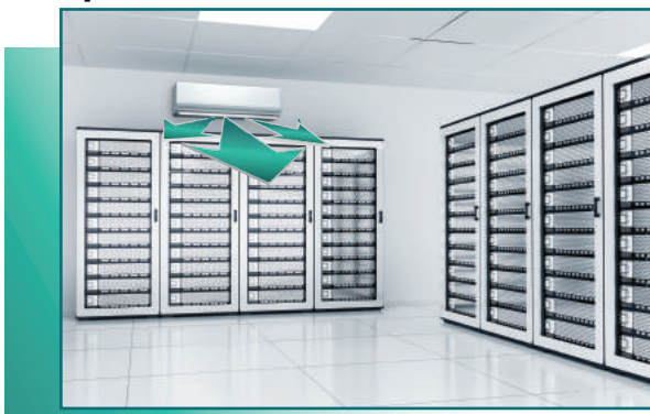
Computer Server Rooms
